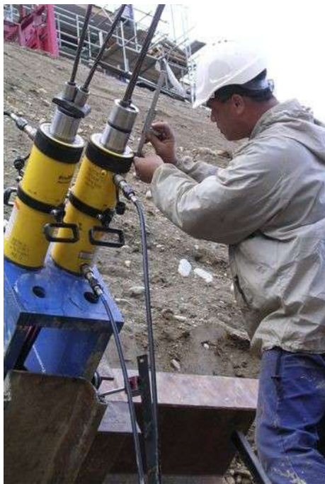
Plate 2. Sacrificial testing of the dual-tendon, actively stressed soil nail prior to excavation. Note proximity of adjacent high level development which will be undercut by 14m face.
